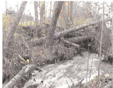
Figure 3 Increased volume of discharge can result in erosion of streambeds and banks (DEP 2005)
